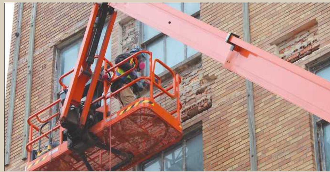
A BRICK SECTION of the east wall of the 150 Bagley building in Detroit is opened up by mason Andrew Kliffel of Bricklayers and Allied Craftworkers Local 2. Employed by Pullman Mason Contractors, he was preparing for the installation of a buckhoist as rehabilitation starts to ramp up on the building.
